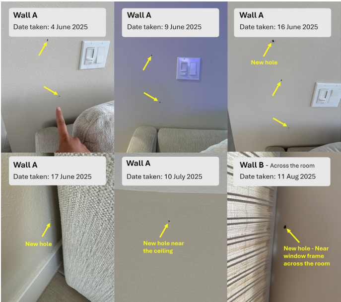
Figure 2. Exit holes detected on the indoor walls of a residential unit in 2025 created by the new house borer [ Arhopalus productus (LeConte, 1850) (Coleoptera: Cerambycidae)]. Each arrow points to the location of an emergence hole.
